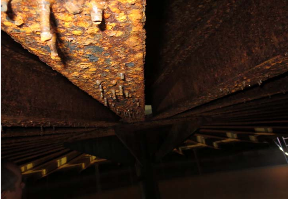
Figure 3: Stalactites Developing on Bottom Flange of Rafter
