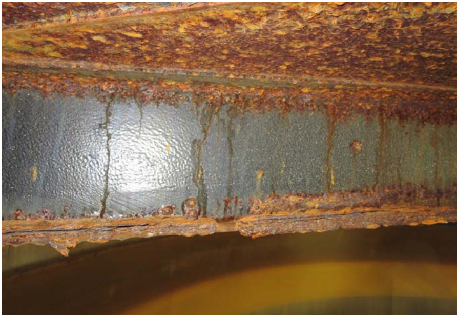
Figure 2: Bottom Flange Corrosion and Section Loss in Rafter
