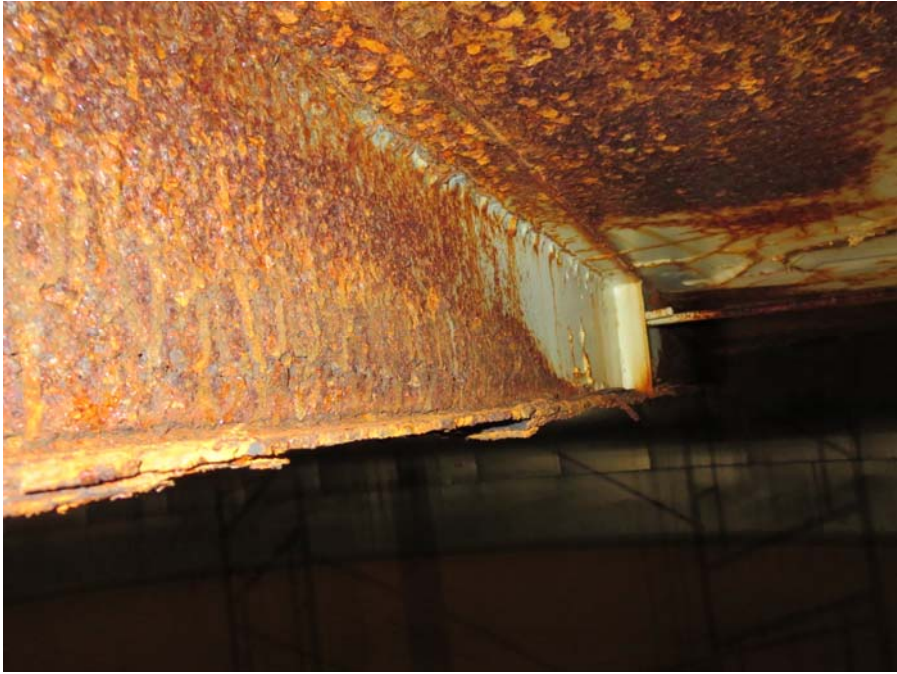
Figure 1: Bottom Flange Corrosion and Section Loss in Rafter
