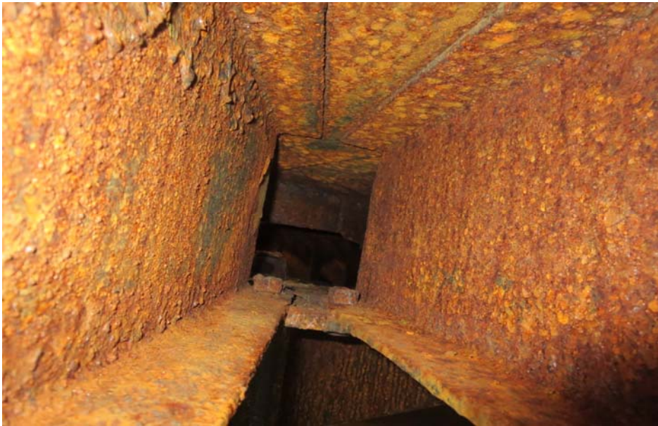
Figure 4: Dollar Plate Corrosion
