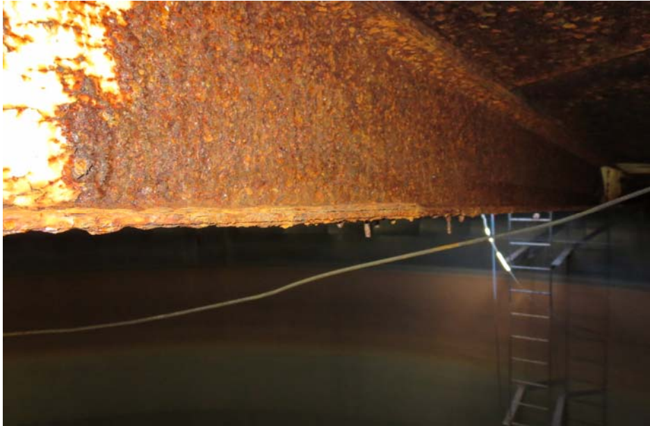
Figure 3: Top Flange Corrosion
