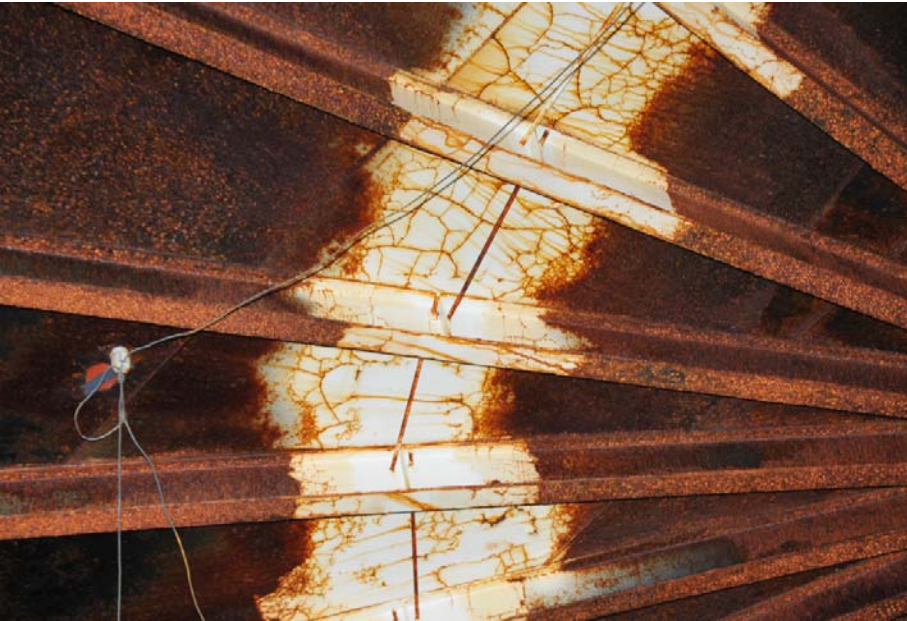
Figure 6: Corrosion on underside of Rafters and Roof Plate
