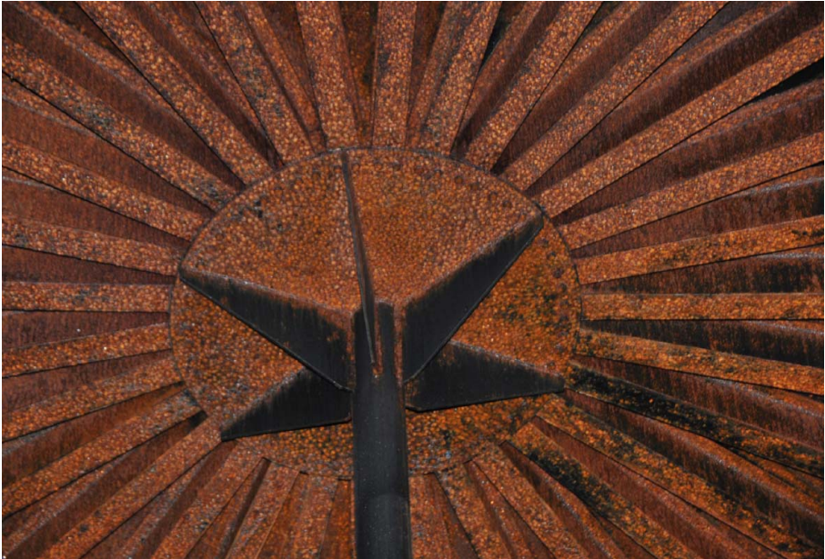
Figure 5: Corrosion on underside of Dollar Plate
