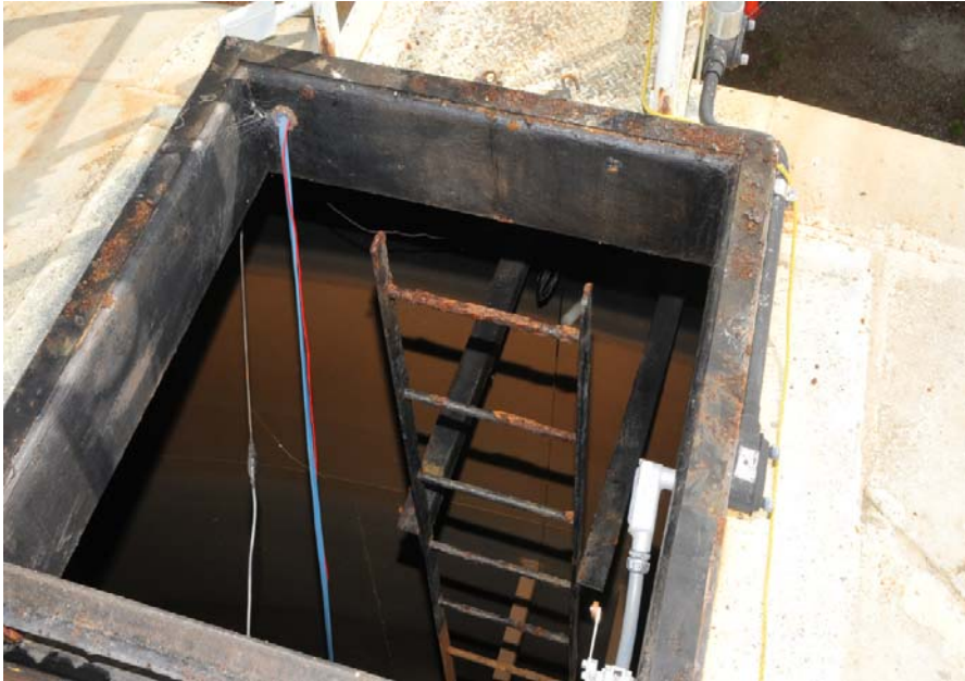
Figure 3: Rusted Ladder on Interior of the Tank
