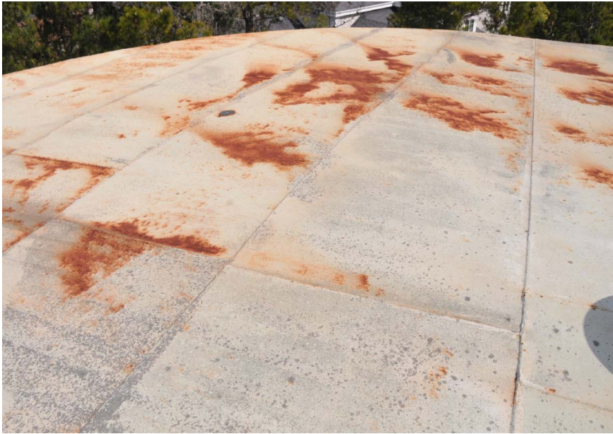
Figure 4: Patches of Rust on the Roof Plate
