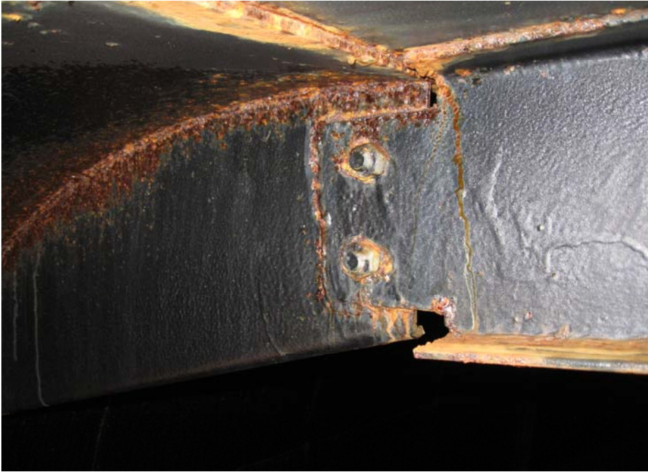
Figure 7: Corrosion on Knuckle Plate
